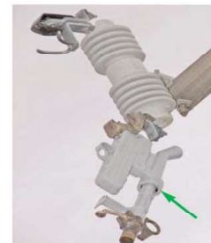
S&C Fault Tamer Fuse - Open
